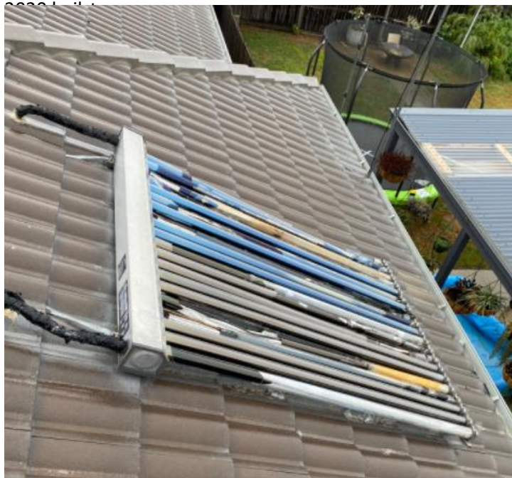
Figure 8: Evacuated tubes damaged by Canberra's January
