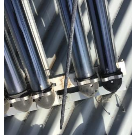
Figure 7: Another example of split copper in solar
